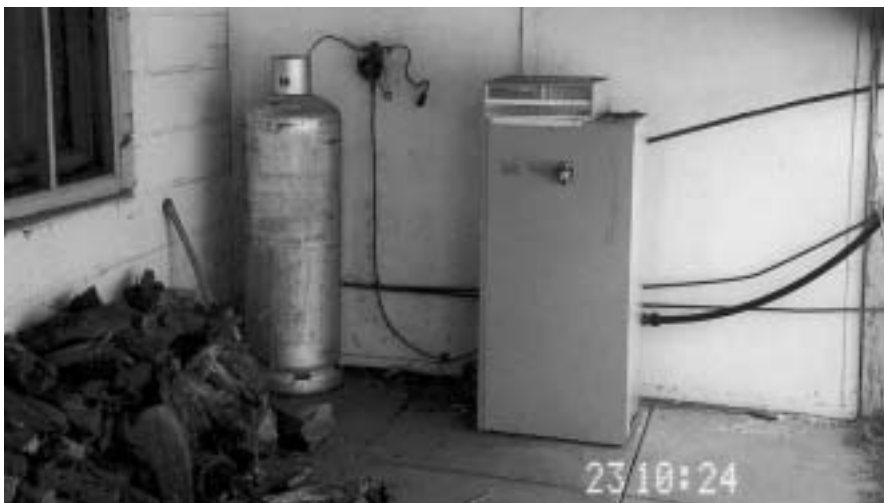
A non-compliant water heater installation that will require rectification work to be carried out
