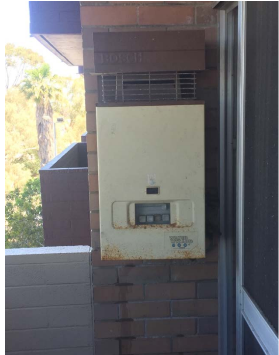
Original non-compliant water heater
