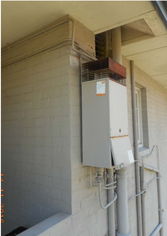
Original non-compliant water heater
