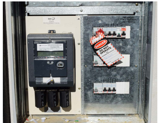
Danger tag on the main switch
