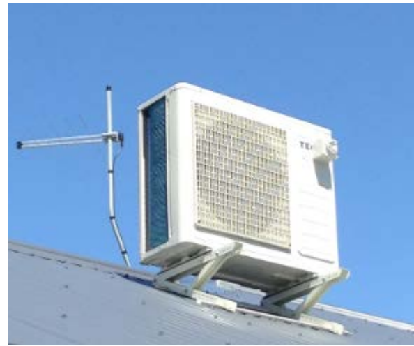
Incorrectly mounted isolator switch fitted to the panel of the external airconditioning unit
