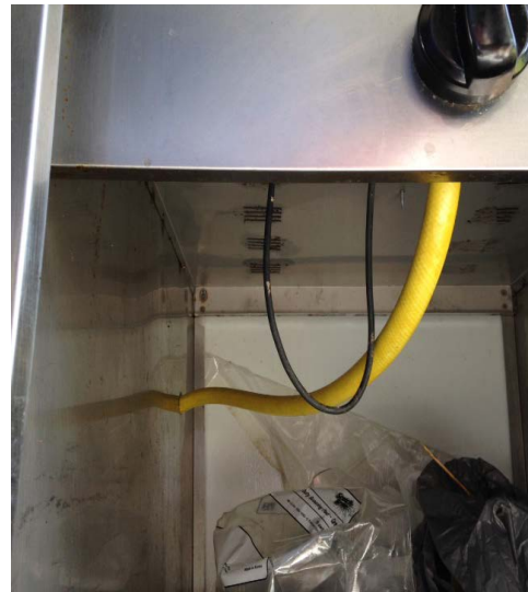
Hose passing through a stainless steel partition
