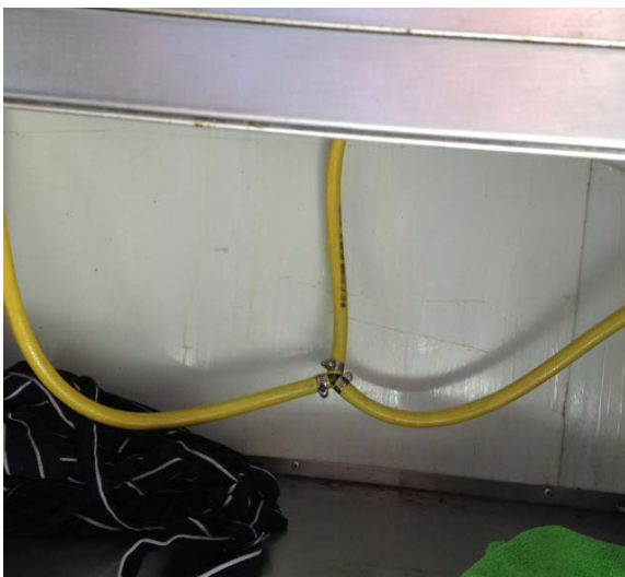
Gas hoses secured with hose clamps
