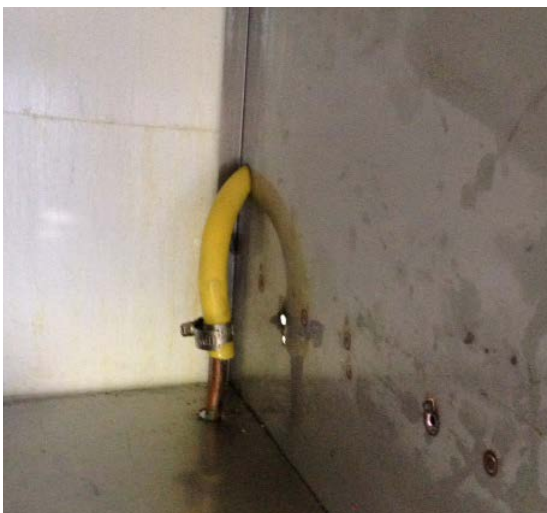
Flexible pipe secured with a hose clamp
