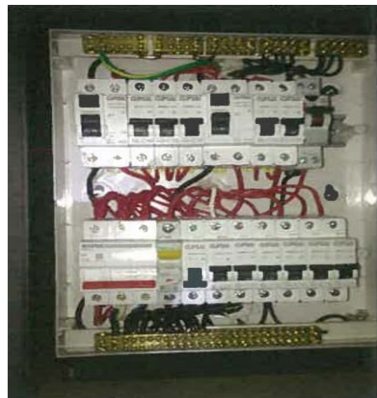
The main switchboard with no MEN connection
