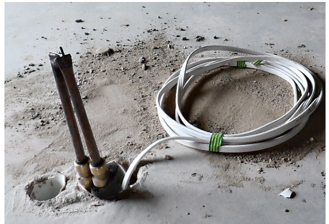
Photo 4: Minimum 100mm separation required between water services and electrical cable.
