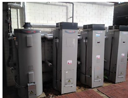
Left hand side internal water heater installed outdoors
