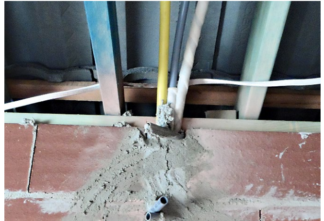
Photo 2: Minimum 100mm separation required between the heated water service (middle grey pipe) and gas (yellow pipe). Minimum separation of 100mm is required between heated water service pipe and electrical cables. Minimum 25mm separation between the electrical cable and the gas service pipes.
