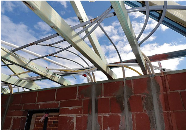
Photo 1: Minimum of 25mm separation required between cold water services, gas pipes and electrical cables. 100mm minimum separation required between heated water services, gas pipes and electrical cables.
