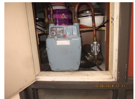
Meter in a combustible box and under kitchen bench
