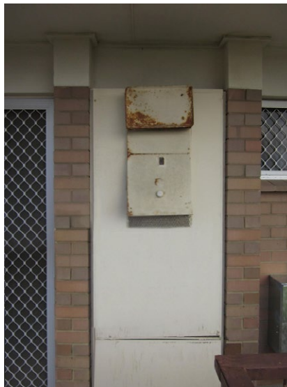
Original water heater locations
