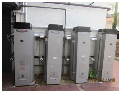
Internal water heater replaced with outdoor unit
