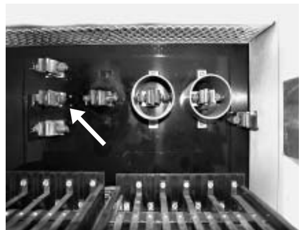
Heat damage causes tension springs to fail
