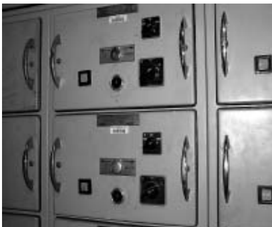
The type of switchboard that is subject to this electrical safety warning
